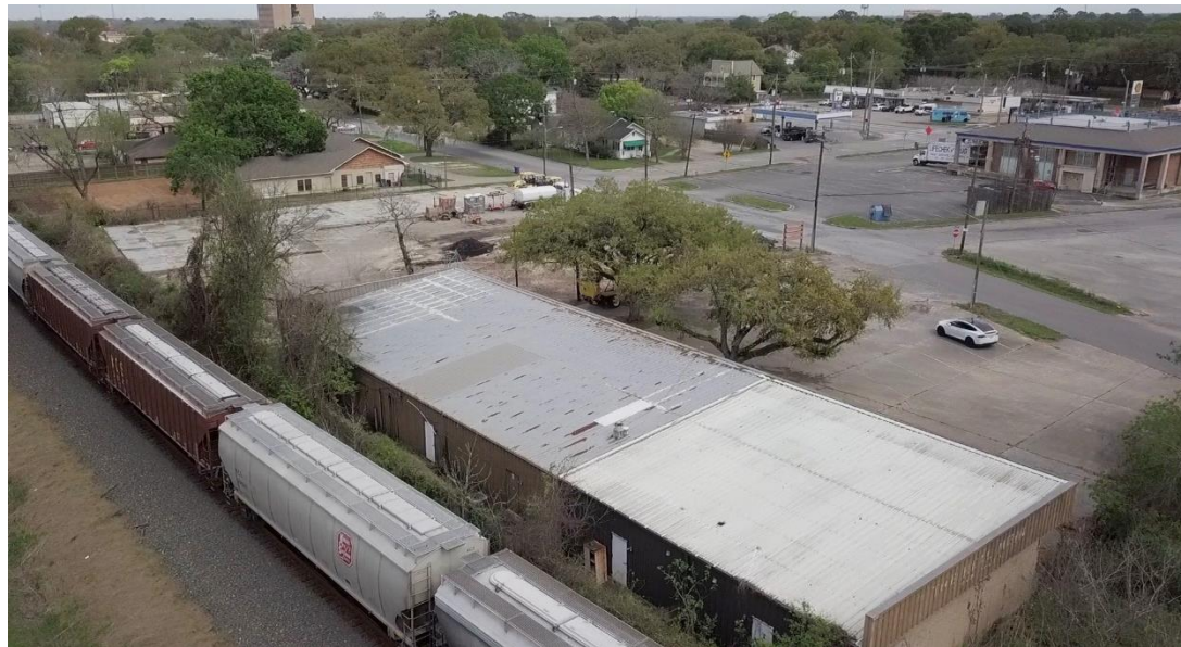
Poor Roof Condition- Adjacent to Active Railroad, Constant Noise Disturbance
