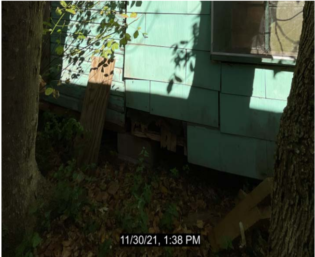
Westside of house. Where two beams meet each other resting on the pier one is decayed and rotten and the other is only sitting on the beam about an inch.
