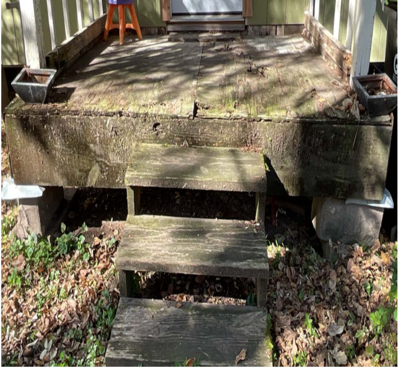
Porch facing Burnet Street is rotten and unstable.
