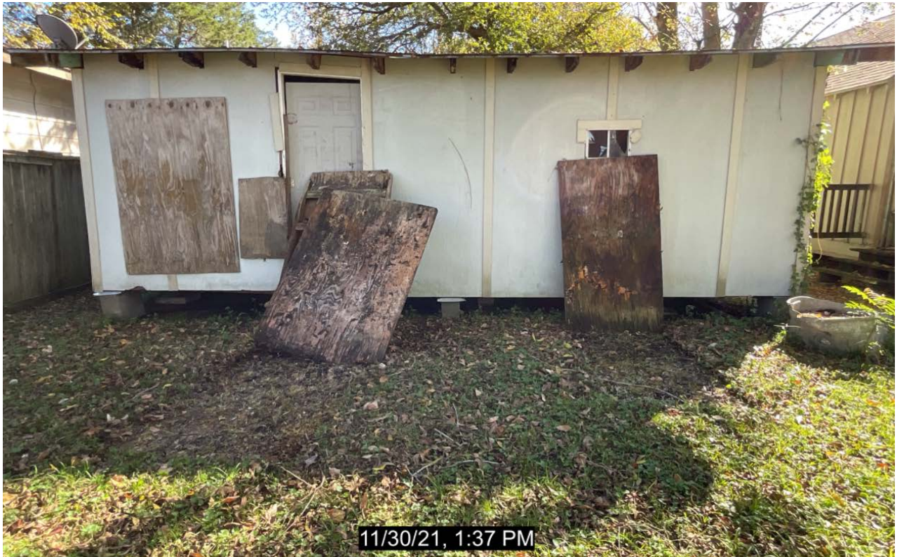
Backside of house / Roof showing signs of sagging
