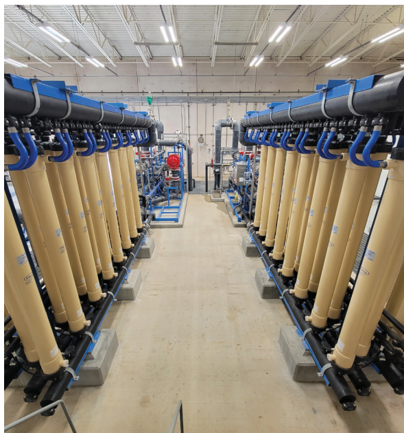
Surface Water Treatment Plant Microfiltration Membranes
